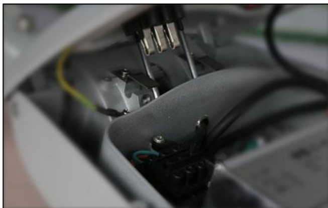
A circuit breaker cuts off the power supply as soon as the luminaire cover is opened, allowing the operator to work safely
